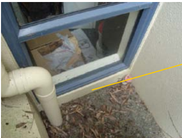
The finished concrete path height has compromised the ground clearance here.
