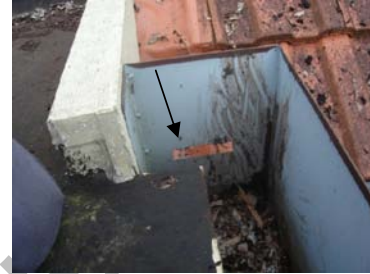
Enlarge the over flow provision to expel collected water from a lower level is required.
