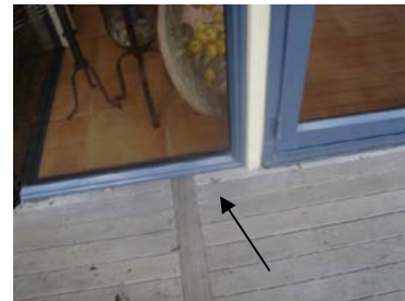
Clearance of 50mm is recommended between the decking against the exterior cladding here.
