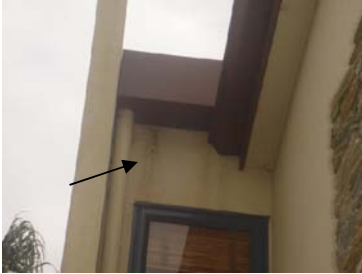
Evidence to suggest excessive water flows beneath the rain head is visible here.
