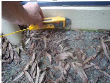
'Search Mode' readings were high. Moisture ingress due to the ground clearance breach is suspected.
